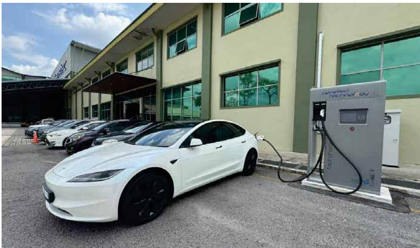
EV Charging Station in EPIC
